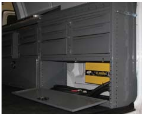
The inverter is installed safely and securely within a locking utility cabinet.
